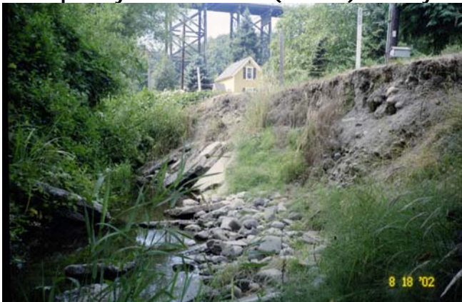
A completely unstable bank (Class 1): Valley 0.4; note the failed revetment.
